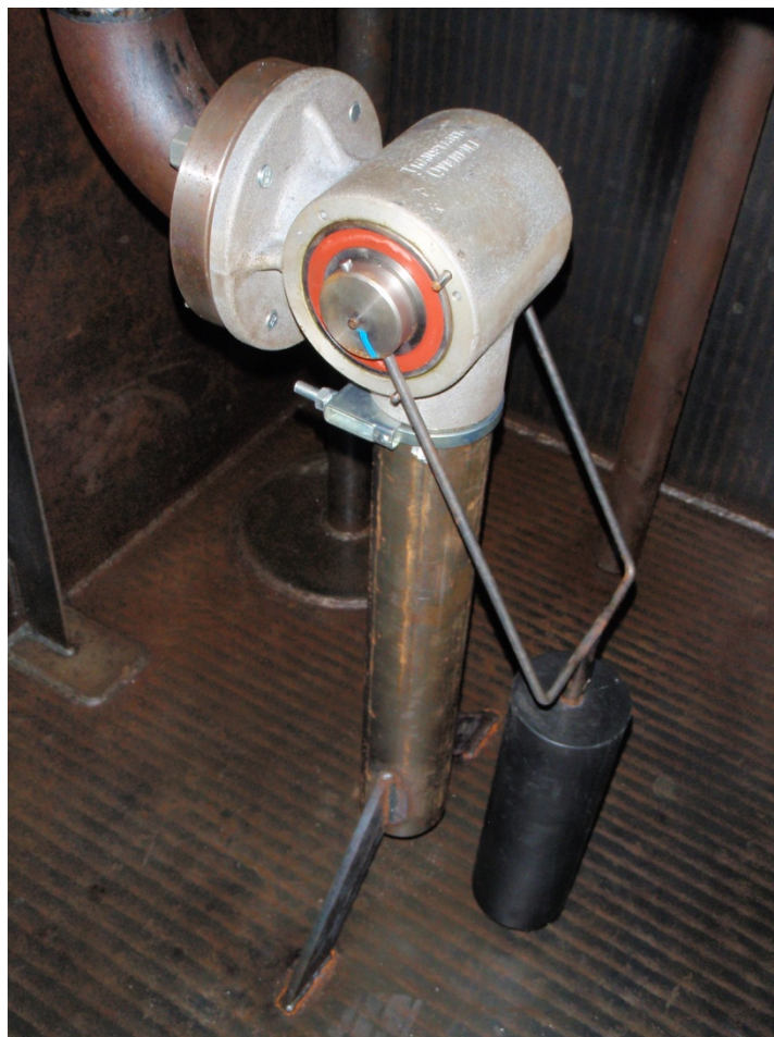
Inside of a Transtank unit showing Overfill Protection Valve
